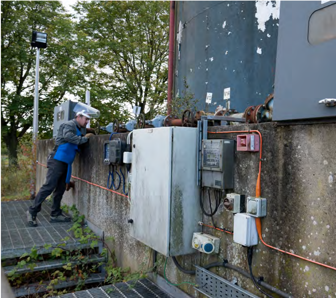
Image 15. Hazards in this image include bulk fuel, high voltage power and an enclosed water tank. Note that the operator's visor has been temporary lifted to aid in visual observation
