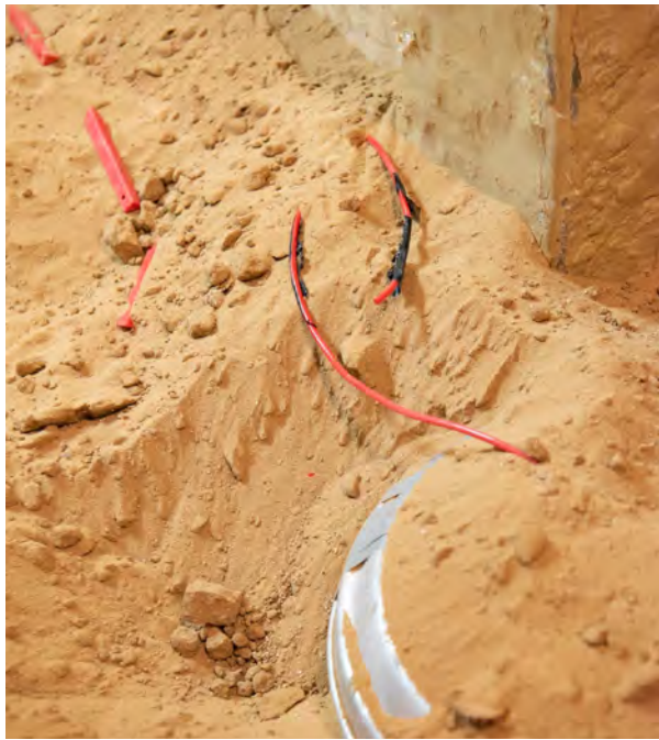
Image 13. Junction separated with enough distance (>10 cm) between the strands of detonating cord to prevent a detonation from propagating
