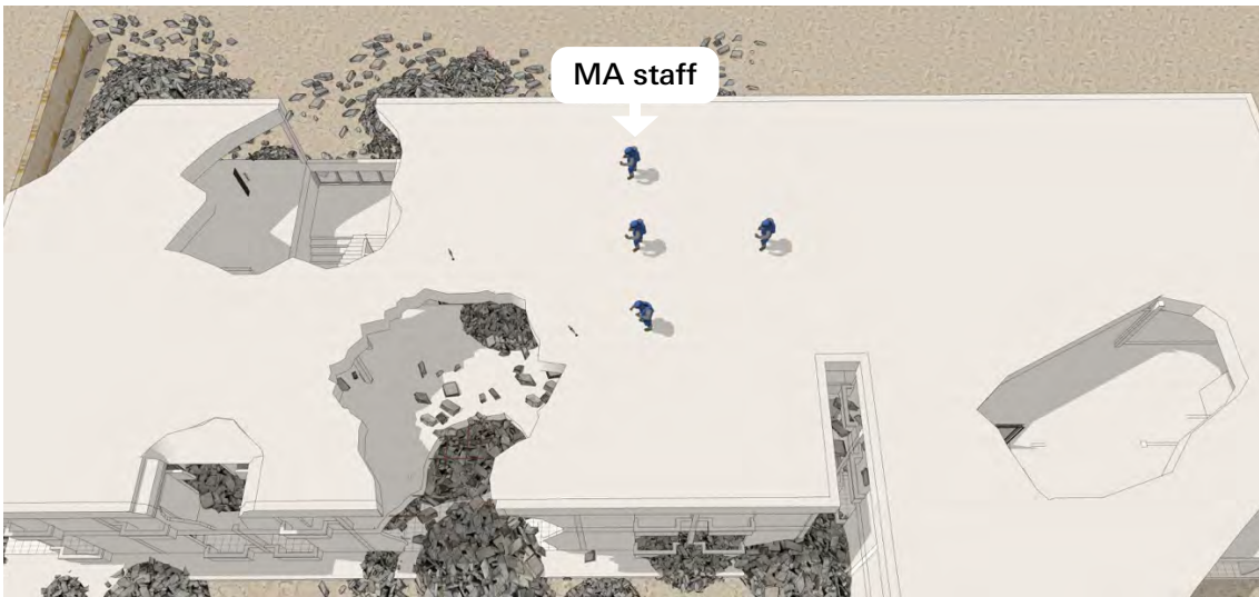
Image 20. Image showing MA staff working at height conducting battlefield area clearance (BAC). Just looking at the damage to this structure, is it safe?
