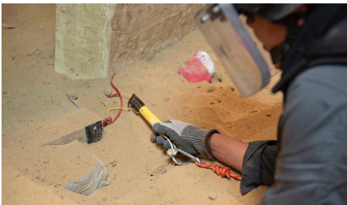
Image 20. Placing semi-remote cutter against single detonator lead. (Red cable is a strop)
