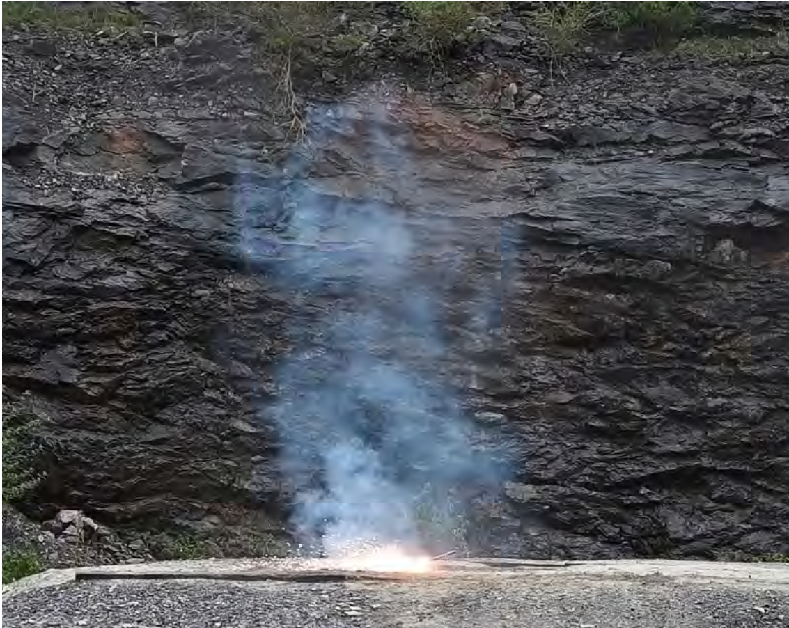
Image 1. Using a pyrotechnic torch / thermite lance on a main charge containing HME
