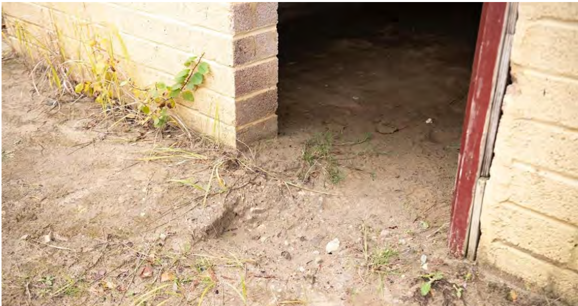
Image 71. Soft conditions can still occur in buildings
