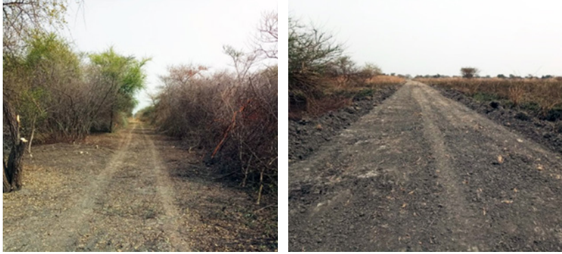
Two sections of Pibor-Akobo Road after being opened by clearance teams (left) and repaired by UNMISS engineers from ROK HMEC (right). © Courtesy of UNMAS
