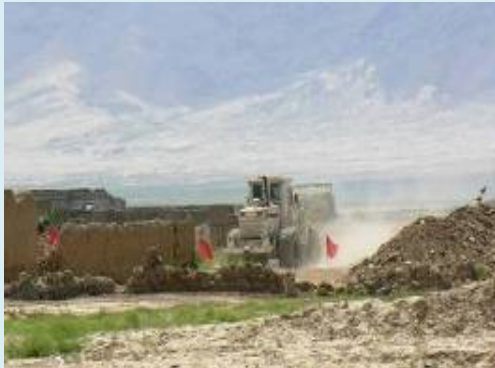
Before: mechanical clearance
