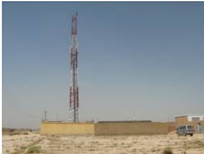
Mobile phone mast on cleared land
