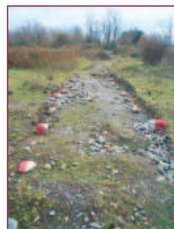
Fig. 2. Ground conditions along the Gumista river.
