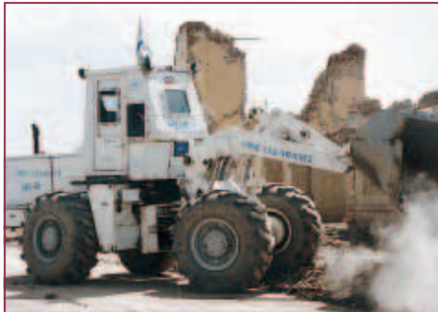
Fig. 17. Converted (armoured) Russian RABA front-end loader conducting rubble clearance, The HALO Trust, Kabul, 1998.
