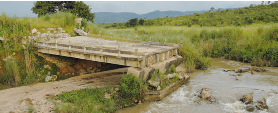
A bridge in need of reconstruction
