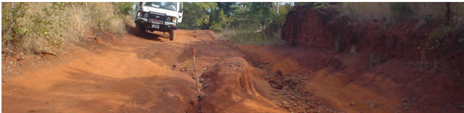
A degraded road
